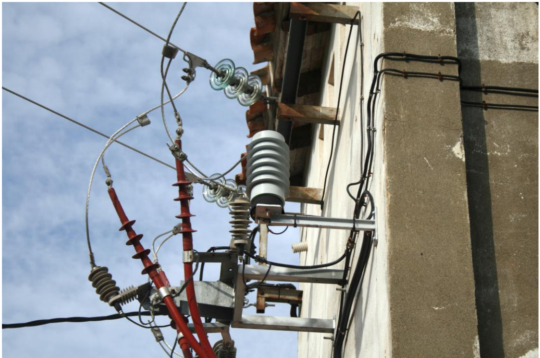
Figure 9 Example of installation of the CAMS-10/RC in overhead line
