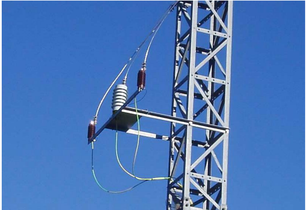
Figure 8 Example of fitting attached to the electrical tower
