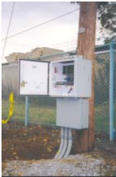
Figure 10: Communication and Power Supply Cabinet
