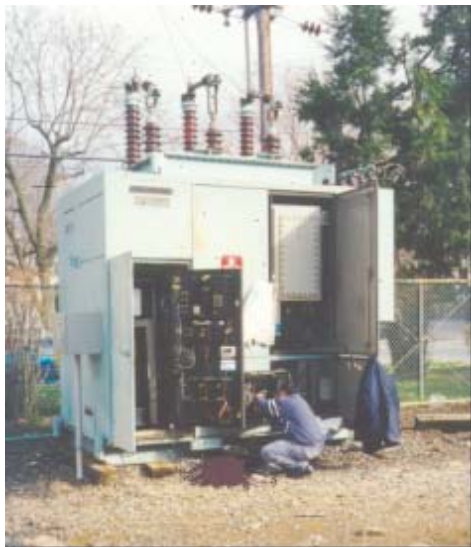
Figure 3: Unit Substation With Added External Control Cabinet
