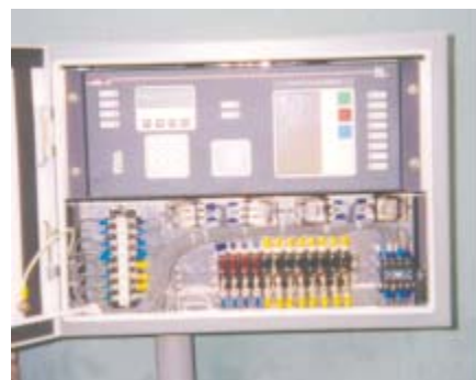
Figure 5: 7IRD Terminal Unit and Test Switches
